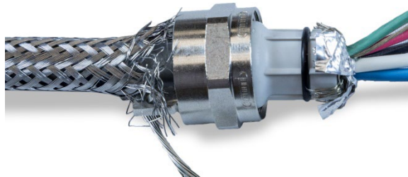
Figure A-44: Inner Braided Shield Wires and Foil Trimmed to Length and Folded Back Over Grommet
