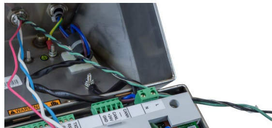
Figure A-52: Grounding Wires and Inner Drain Wire Twisted Together
