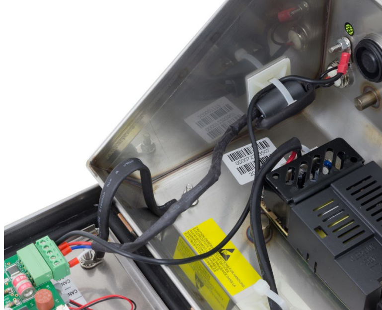
Figure A-56: PowerDeck Connector Installed in the IND246 POWERCELL
