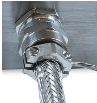
Figure A-47: Cable and Cable Gland Installed in Enclosure
