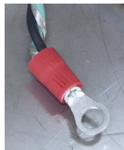
Figure A-53: Ground Wire Termination
